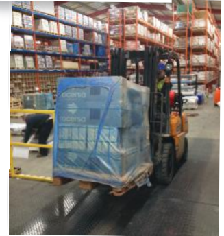
Dock levelling system, Cardiff
