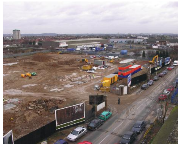
Above: New site purchased - Development of new head office at Chadwell Heath Right: Under construction - New head office at Chadwell Heath
